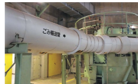
廃棄物空気輸送管 Pneumatic trash-carrying ducts
